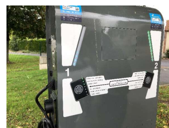
Borne de recharge double 12kW/h
